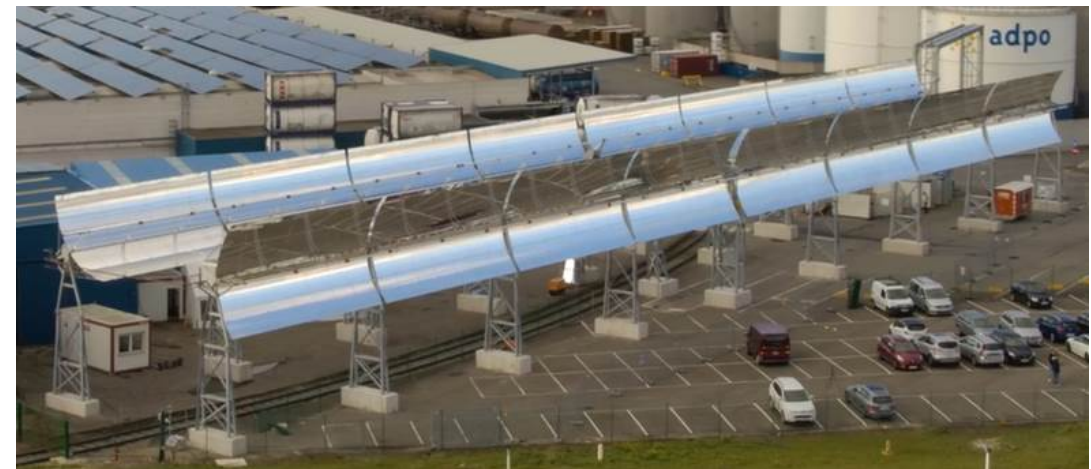
Parabolrinnenfeld Foto: Solarlite CSP Technology GmbH
